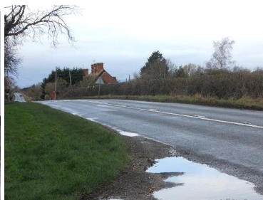
Verge damage, B4077
